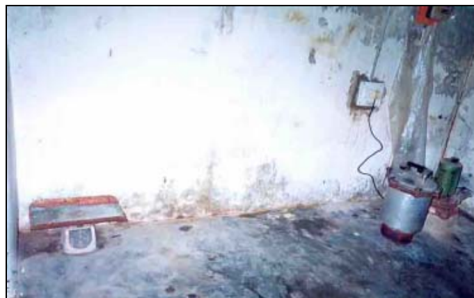
Figure 5 - Labour room of one of the PHC visited. A baby weighing machine and autoclave which was not being used were kept in the floor in two corners of the labour room. The floor is dirty and there is no other equipment or labour table.
